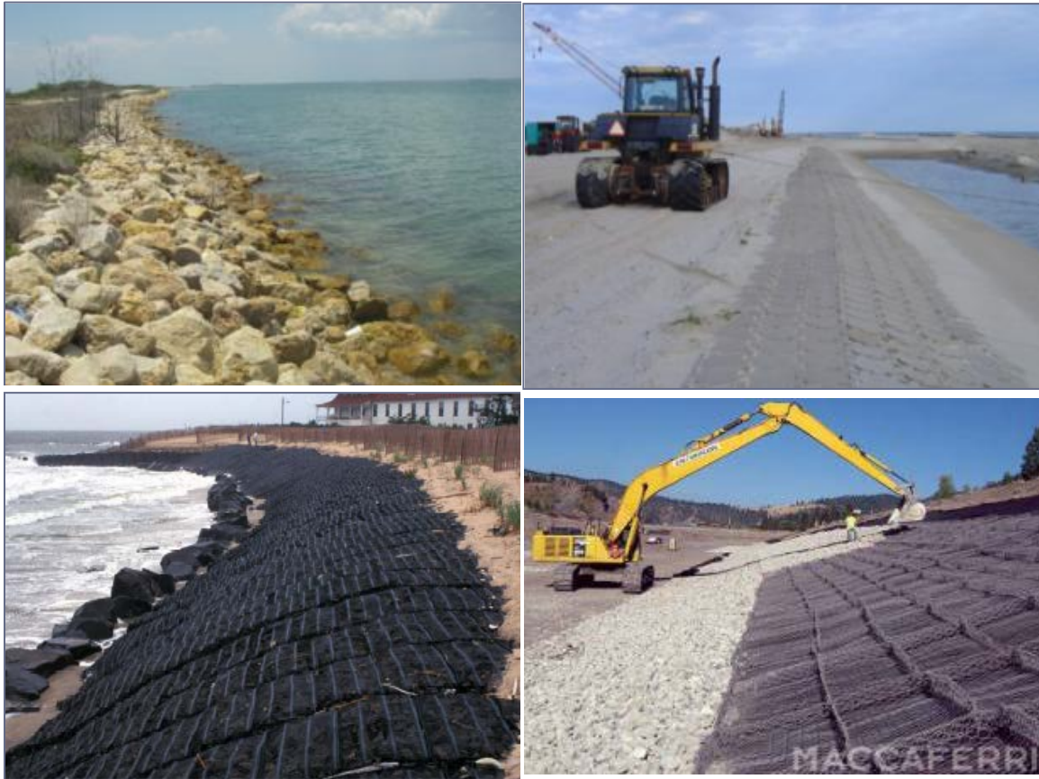
Figure 34. Examples of Revetment Structures: Quarry-stone (upper left), ABM (upper right), marine mattress (lower left), and gabion (lower right) (courtesy of Maccaferri)
