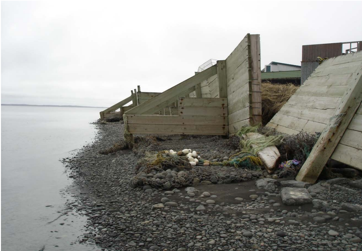
Figure 19. Broken Section of Wooden Seawall
