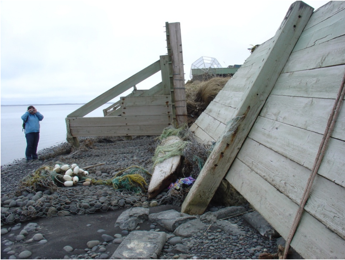
Figure 17. Undermining and Removal of Material behind a Portion of the Timber Sea Wall in the Southeastern Portion of the Community
