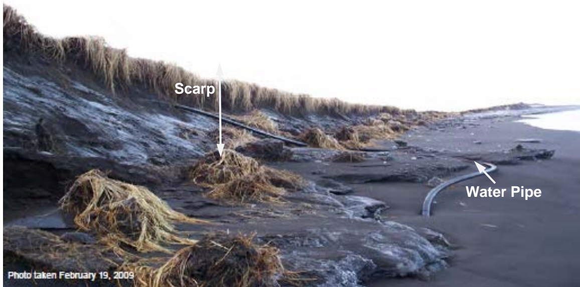
Figure 29. Bering Sea Shoreline Erosion (HDR 2010b; Notice exposed water transmission pipe)
