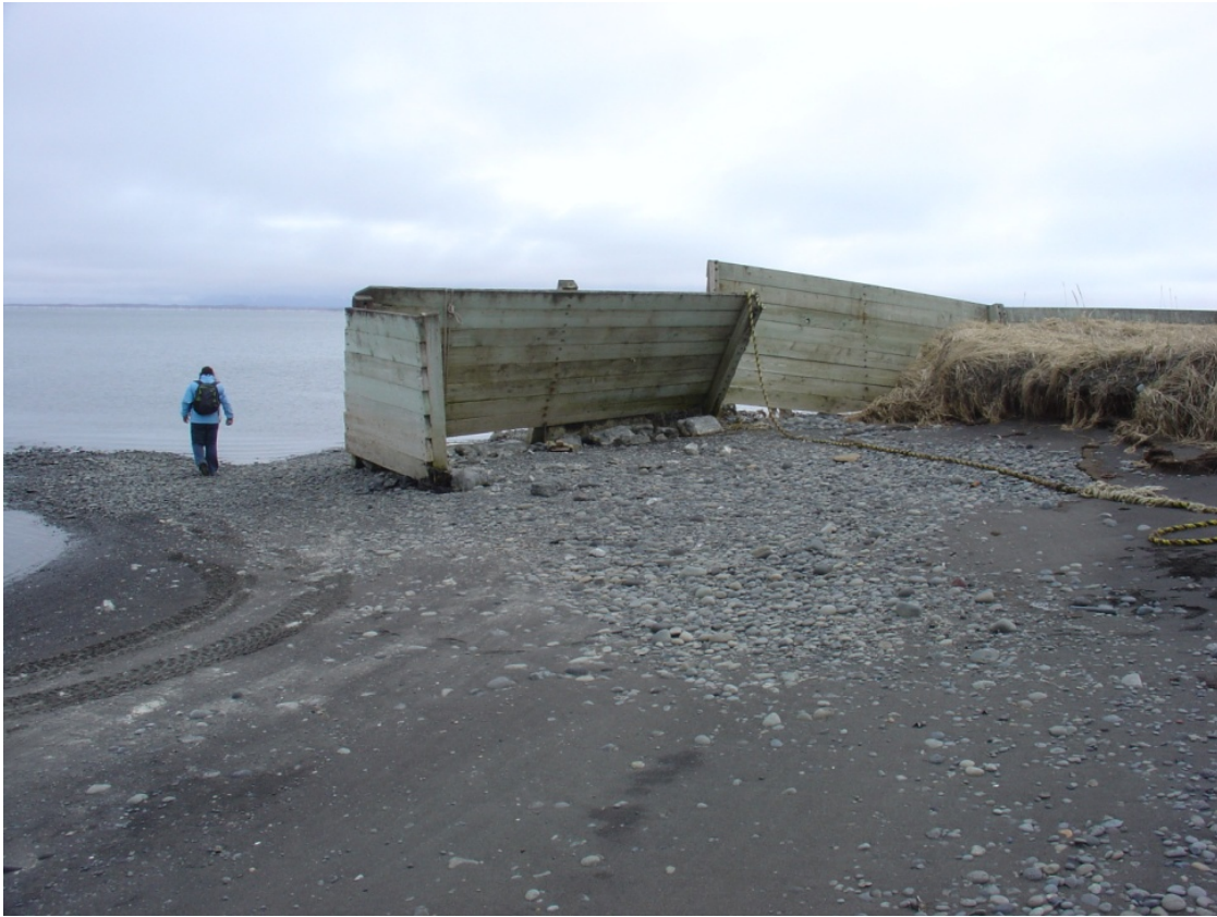
Figure 20. Severe Erosion of Wooden Sea Wall on Eastern End of the Wall
