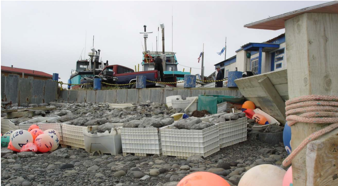
Figure 23. Rock-Filled Fish Totes Used to Reinforce the Wooden Seawall
