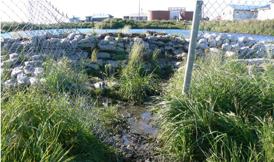
Photo 6. Leaking sewage lagoon next to school and subsistence fish drying areas.
