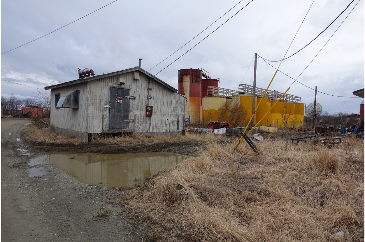
Figure 6. LKSD fuel electric power infrastructure. May 11, 2018
