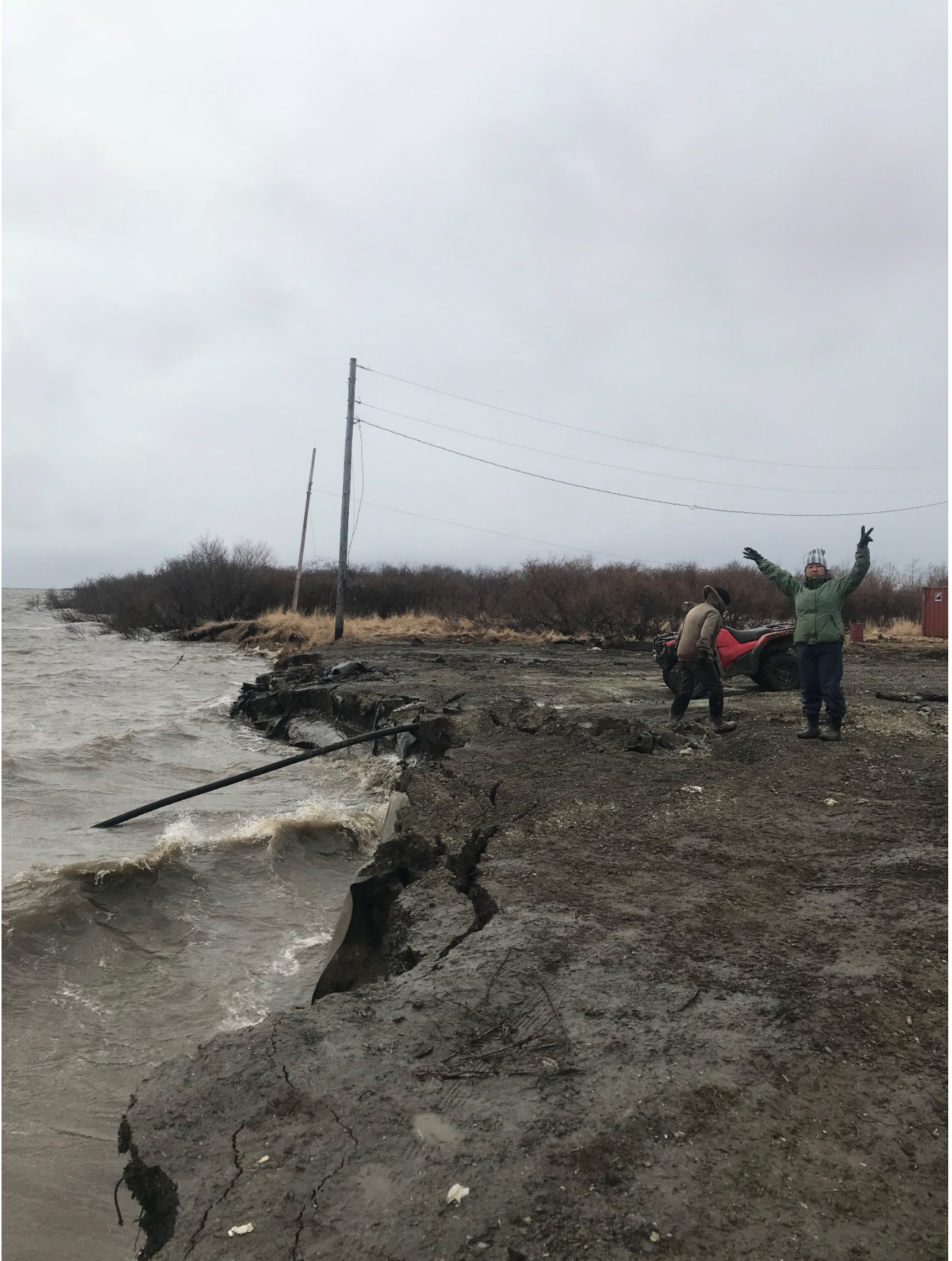
Figure 4. Erosion during May 12-13, 2018 storm event. Taken May 13, 2018. Credit: Mike Black.
