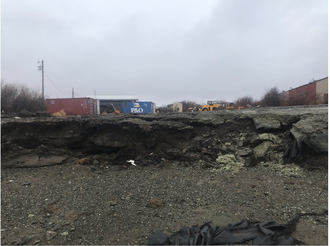
Figure 3. May 13, 2018 storm damage. Note the close proximity to the Napakiak school (right). Credit: Mike Black.
