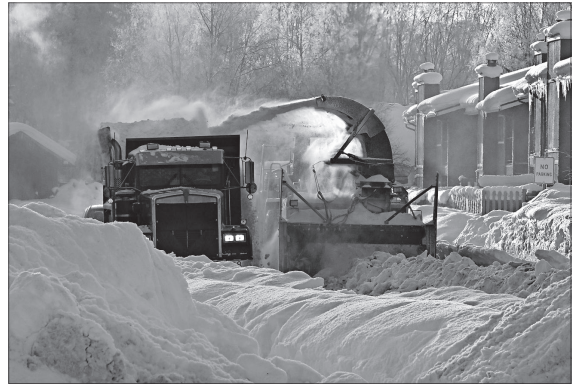
A snow removal and street-widening operation on Pioneer Drive in Muldoon on Wednesday.
